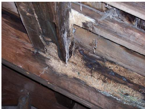
Figure 12. Advanced fungi decay.
