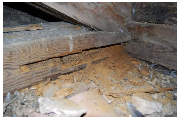
Figure 13. Deep damage caused by insects in the rafter ties.
