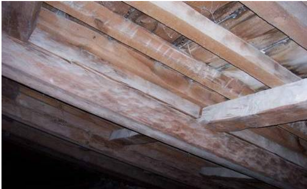
Figure 8. Longitudinal splitting in the rafter.
