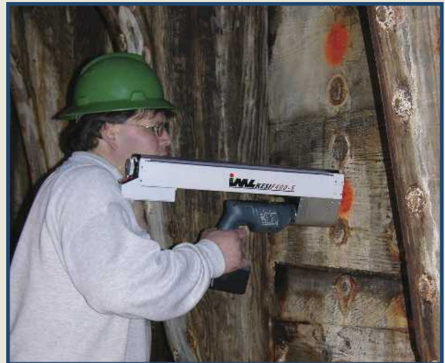
Figure 2. — Field inspection using a resistance drilling device to locate areas of deterioration.
