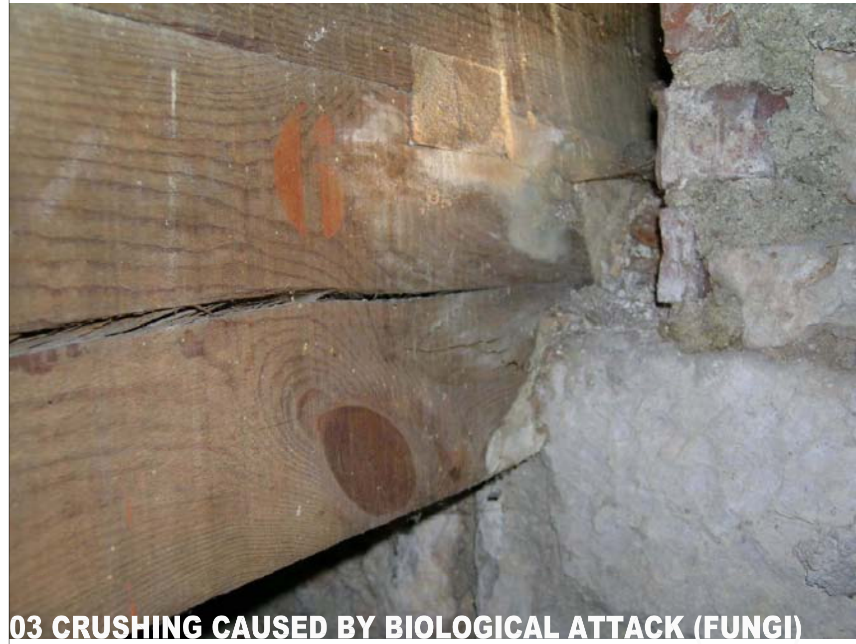
03 CRUSHING CAUSED BY BIOLOGICAL ATTACK (FUNGI)
