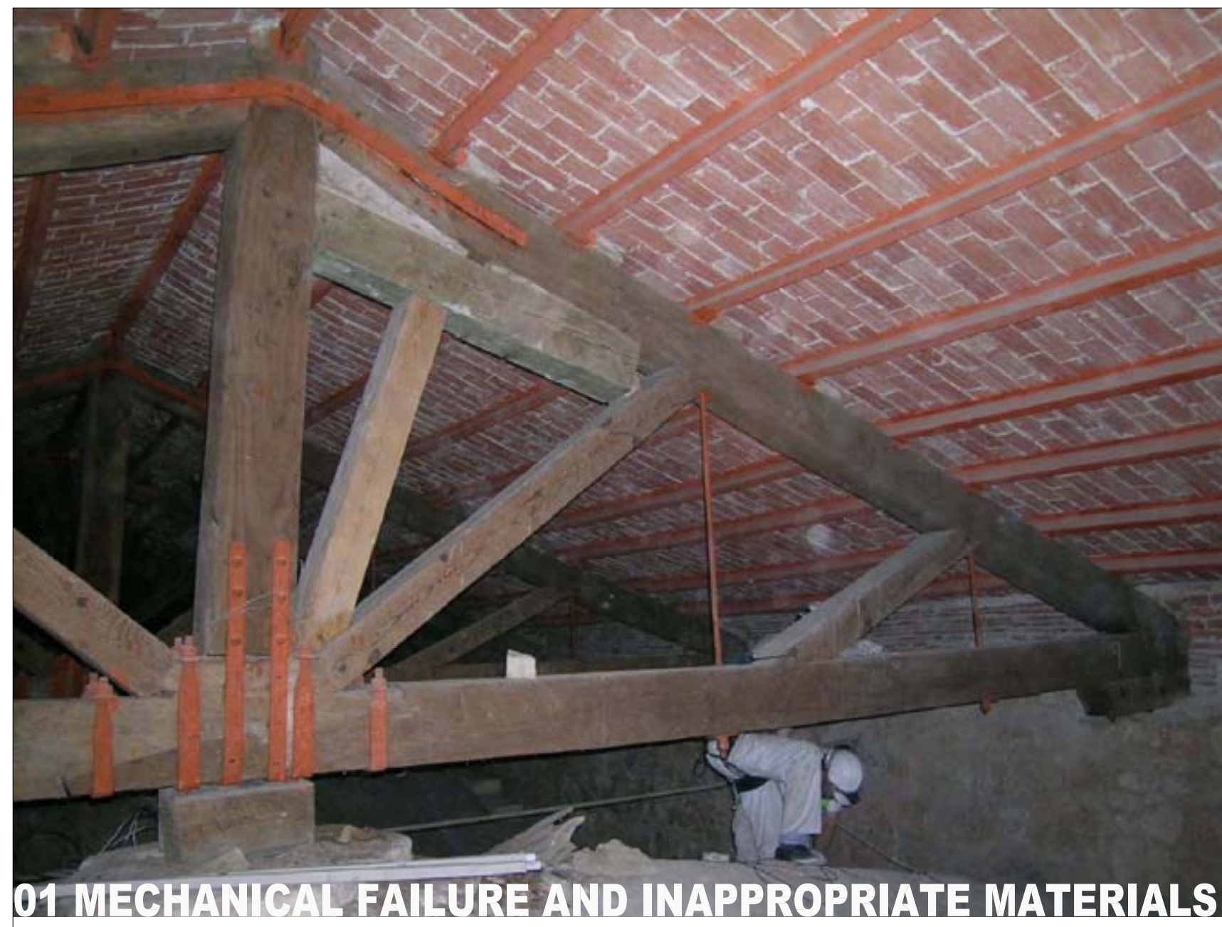
01 MECHANICAL FAILURE AND INAPPROPRIATE MATERIALS
