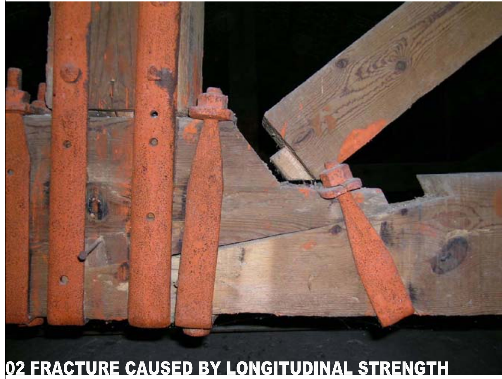
02 FRACTURE CAUSED BY LONGITUDINAL STRESS
